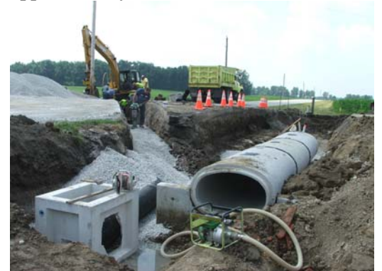
Prolonged flooding at the intersection of Hardin Pike and SR# 219 was eliminated. A new elliptical overflow pipe, the replacement of a subsurface tile with catch basins and an outlet waterway was jointly installed by this department and ODOT forces.
