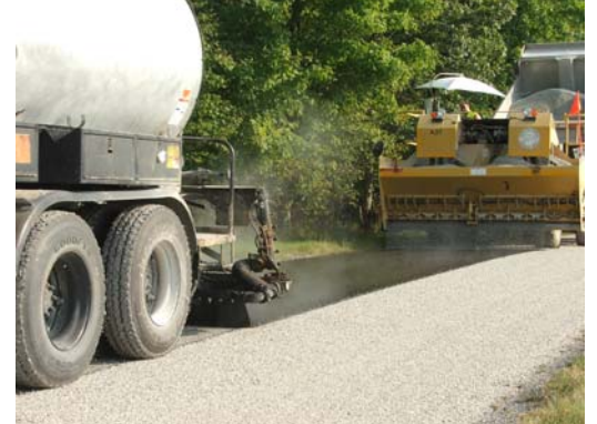
The above photo shows the tar distributor applying the 160° liquid asphalt emulsion at a rate of 0.40 gallons per square yard followed immediately by the chip-spreader placing 24# of limestone per square yard. The rubber tired roller then follows close behind "seating" the stone into the asphalt before it cools. This preventive maintenance measure provides a new wearing surface over the oxidized pavement, and fills the reflective cracks for approximately 1/5 th the cost of new hotmix.
