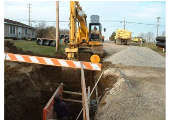
Crews replaced a century old 18" subsurface clay tile along the south side of Lock Two Road east of SR# 66, with a 24" diameter plastic pipe early in the spring. The use of a trenchbox and shorter sections of pipe were required due to the 10' depths.
