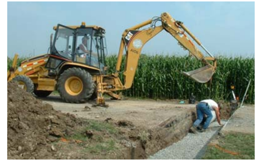
During 2007 our crews replaced drainage culverts (above) crossing under the highways at 51 locations. All but three of these installations were completed and opened to traffic in less than one working day.
