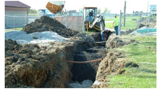
County Commissioners paid the highway department to extend a 12” diameter sanitary sewer (above photo) at the fairgrounds. The installation was complicated by crossing a myriad of fiber optic communication and gas lines.
