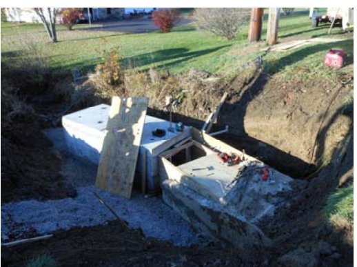
CR#33A is being programmed to receive federal funding for resurfacing within the near future. County Crews are currently extending existing culverts (above) to provide needed safety shoulders in anticipation of the upcoming project.
