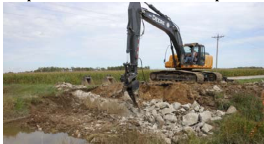
The excavator with the hydraulic demolition hammer (above) was used to remove the existing walls for a new 38' span bridge on National Road over the Grassley Ditch. The broken concrete was then reused as rip-rap for erosion control along the new walls.
