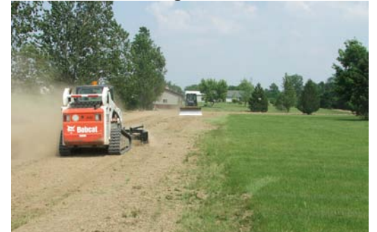
Seeding crews (above) are performing yard repairs to trenches resulting from the new storm sewers installed as a part of the Bryant Ditch petition in Noble Township.
