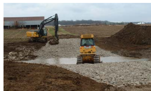
To gain access to several acres of farmground at the Neil Armstrong Airport, the County Commissioners reimbursed our department for replacing an antiquated farm bridge with a “drive-through” crossing (above) using 500 tons of various gradations of stone.
