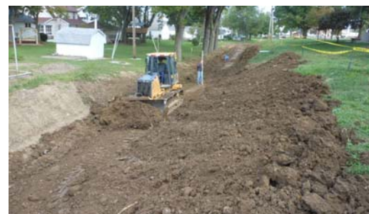
The Village of New Bremen reimbursed the County for the replacement of 600 feet of a century old 18” diameter storm sewer through the park area with 24” smooth walled plastic pipe (above photo). Crews also reshaped the parallel surface drain.
