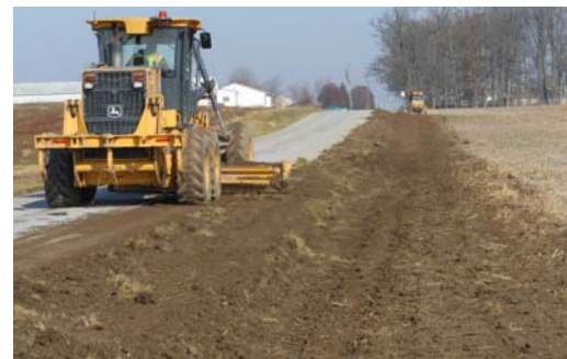
County crews used 507 tons of milled asphalt to widen ½ mile of the Mercer Line (above) by three feet and provide safety shoulders.
