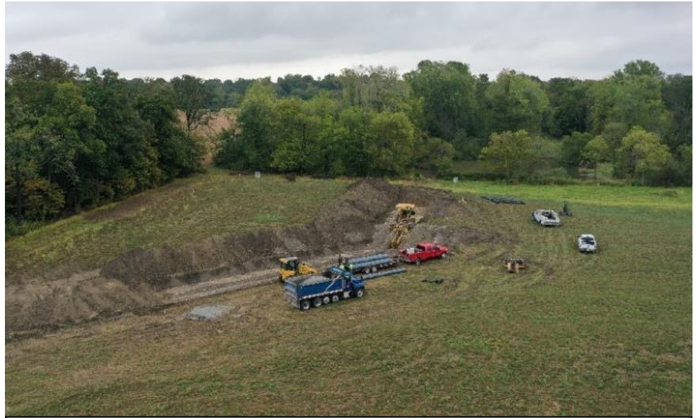
Sand Ridge Excavating scalping dirt for tile installation approximately 9' deep for the Ewald Ditch.
